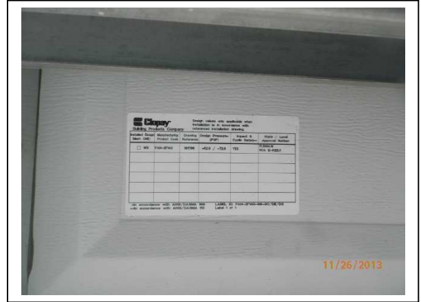
Rated sticker on garage door
