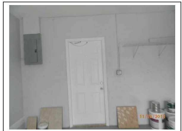
Impacted rated exit door
